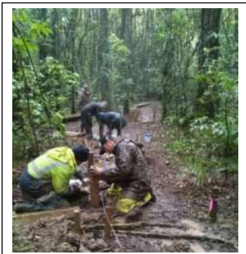
Photo top: checking tunnel cards, 1200, no pest prints! Photo left: Vols from Balance Kapuni dug in 62 posts!
